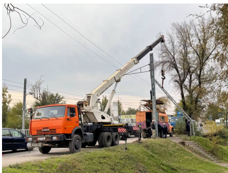
Above: Directly across from the other wrecked pole this one also had collapsed. Various service vehicles are seen in attendance. Line 11 trolleybuses still managed to pass this spot.
